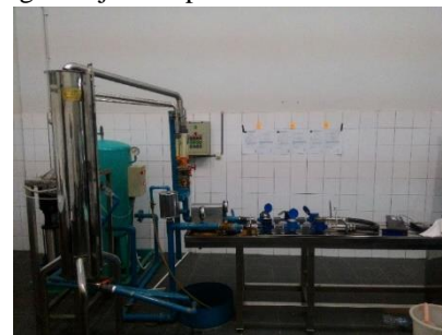
Gambar 1. Instalasi Pengujian Meter Air ( Test Bench Water Meter )
